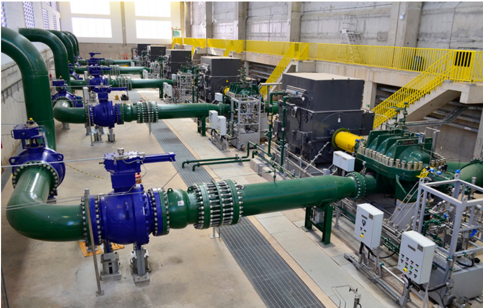
Sulzer has delivered part of a major water scheme in Brazil
