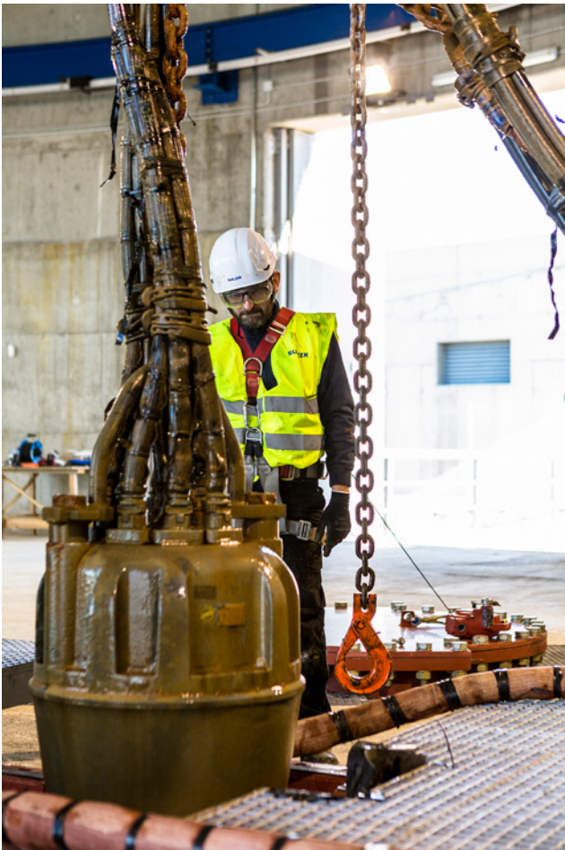
Sulzer delivered a turnkey solution including the infrastructure for removing and installing the pumps for maintenance
