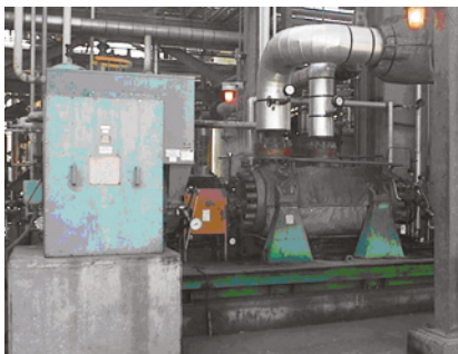
The rerated pump with increased performance operating on site
